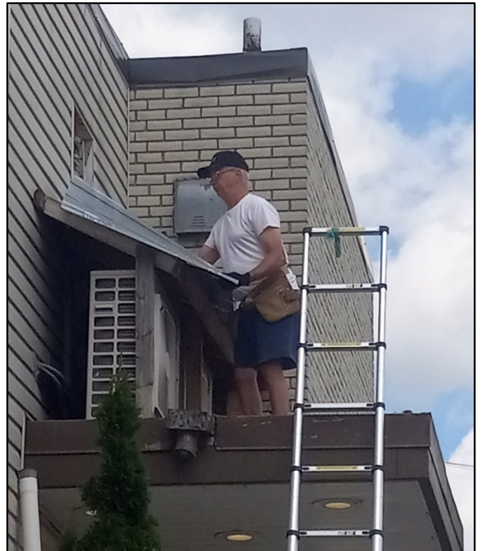
Building Manager Kari Malmstrom was hard at work, seen here removing the small roof covering the two A/C fans to provide access for servicing.
